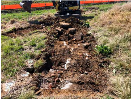
TP07 – large volumes of building demolition waste identified in the area adjacent a creek transecting the site
